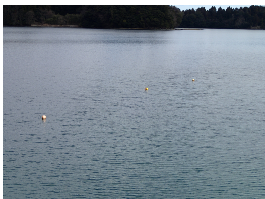
(c) Mark buoys for anchor and connecting shackle, and the floating structure
